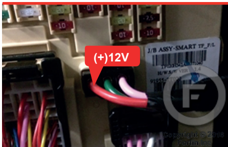
① In the front of the fuse box Boite à fusible
